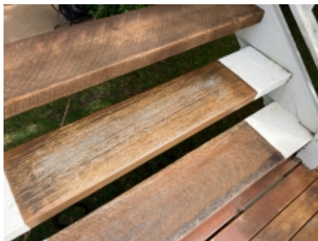
All external timbers should be sealed to prevent decay.
