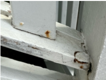
Timbers affected by fungal decay should be repaired to prevent possible timber pest attack. A licensed builder should be engaged for further advise.
