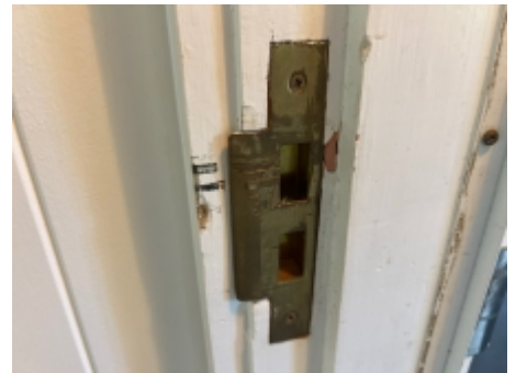
Striker plate needs to be adjusted to allow the door to latch closed.
