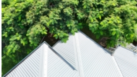
Foliage should be cleared away from all structures.
