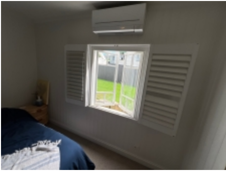
Timber windows require adjusting to allow smooth operation throughout
