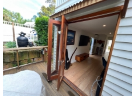
Bifold doors require servicing to allow smooth operation.
