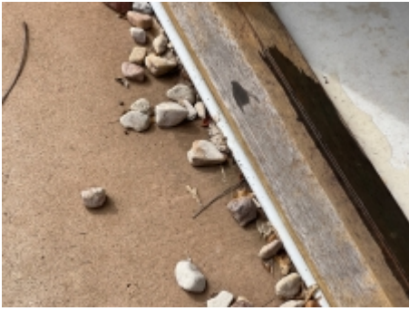
All external timbers should be sealed to prevent decay.
