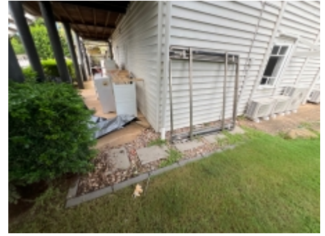
A 75 mm exposed slab edge should be maintained under all external cladding, a pest controller should be engaged for further advice.
