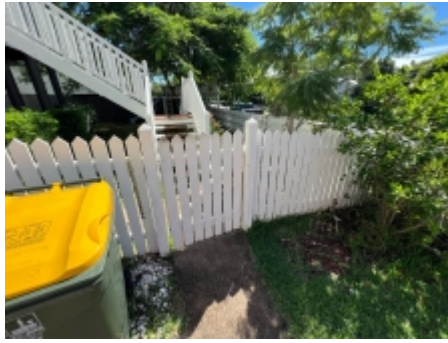
Timber fences are in varying degrees of decay and stability.
