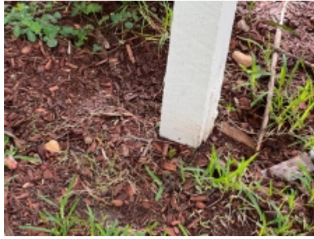
A 75 mm inspection zone should be maintained under all timber building materials where possible. A carpenter should be engaged for further advice.
