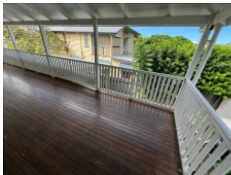
Timbers affected by fungal decay on the stairs and handrails needs to be replaced to prevent possible personal injury. A licensed carpenter should be engaged for further advice.
