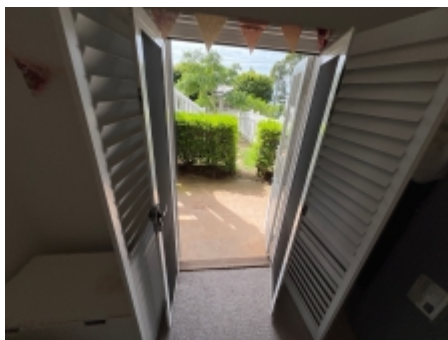
Door needs to be adjusted to allow smooth operation.
