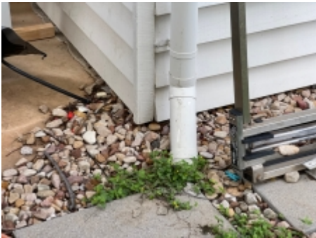
A 75 mm exposed slab edge should be maintained under all external cladding, a pest controller should be engaged for further advice.
