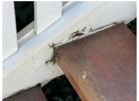
Timbers affected by fungal decay should be repaired to prevent possible timber pest attack. A licensed builder should be engaged for further advise.
