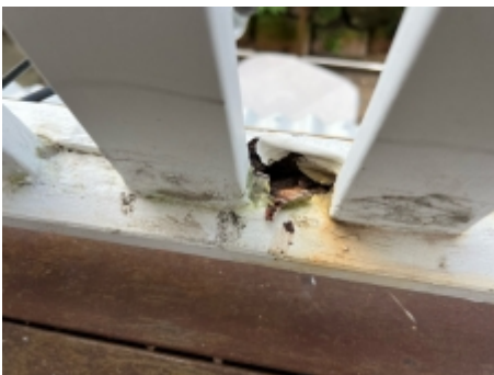
Timbers affected by fungal decay on the stairs and handrails needs to be replaced to prevent possible personal injury. A licensed carpenter should be engaged for further advice.
