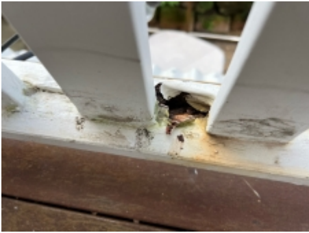
Timbers affected by fungal decay should be repaired to prevent possible timber pest attack. A licensed builder should be engaged for further advise.
