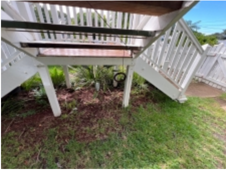
A 75 mm inspection zone should be maintained under all timber building materials where possible. A carpenter should be engaged for further advice.
