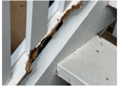
Timbers affected by fungal decay should be repaired to prevent possible timber pest attack. A licensed builder should be engaged for further advise.
