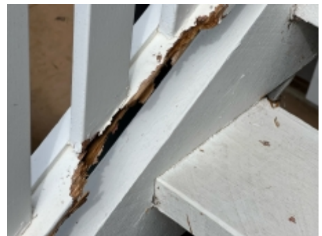
Timbers affected by fungal decay on the stairs and handrails needs to be replaced to prevent possible personal injury. A licensed carpenter should be engaged for further advice.
