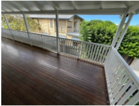
Timbers affected by fungal decay should be repaired to prevent possible timber pest attack. A licensed builder should be engaged for further advise.
