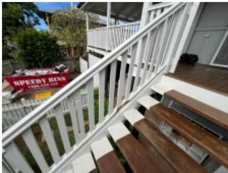
Timbers affected by fungal decay should be repaired to prevent possible timber pest attack. A licensed builder should be engaged for further advise.
