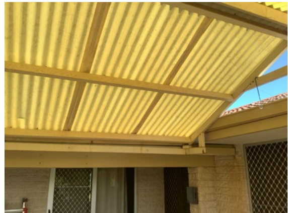
The West elevation Patio structure is connected to the metal fascia of the main residence only which is not designed to take load and has caused sagging and damage to the fascia gutter and eaves. Repairs, modification and/or removal is required to prevent further damage and to make safe.
