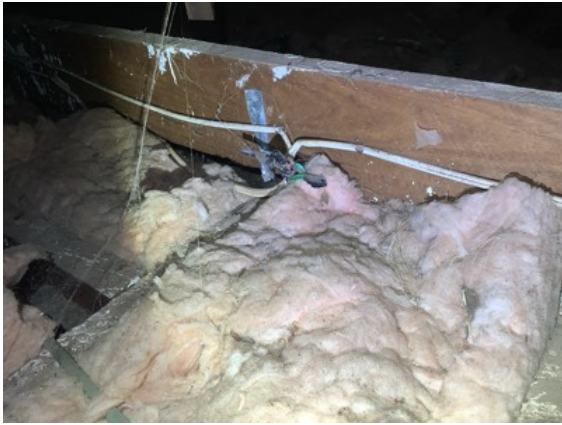
Exposed wiring junctions observed in the roof void above the Kitchen area. Recommend having an Electrician install junction box's at all connections to make safe.
