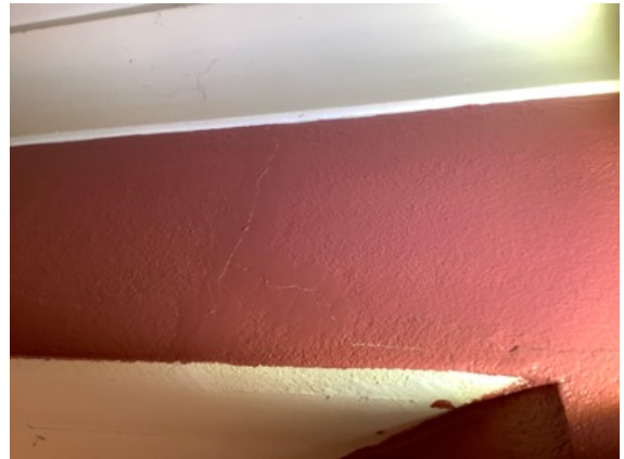
Family - Appearance cracking noted to wall linings at some isolated areas throughout the home. Recommend maintenance/repairs.
