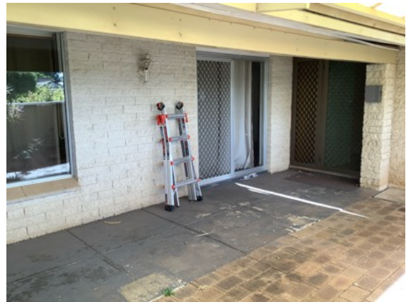
Wood rot damage and significant sagging/deflection noted to the Verandah beam. There are 2x marks on the ground where previous piers or posts appear to have been removed. Recommend invasive inspection and repairs which may require a beam replacement and additional supports installed.
