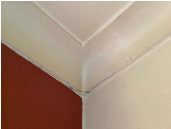
Family - Typical appearance cracking noted to the cornice and wall junctions at some isolated areas throughout the home. Recommend maintenance/repairs.
