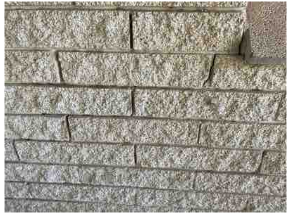
East elevation - Stepped appearance cracking noted to the exterior brick wall below the Activity Room window. Recommend maintenance/repairs and to monitor over time.
