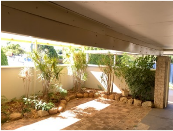
Significant deflection, distortion and sagging noted to the Verandah beam due to inadequate support. Recommend repairs which may require replacing the beam and installation of additional supports.
