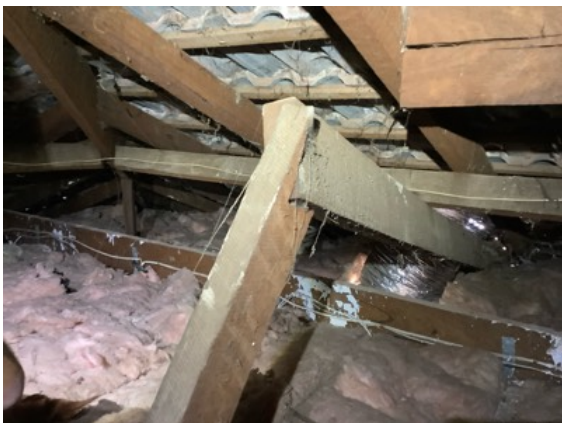
Significant twisting and failed fixings noted to the scissor strut above the Kitchen area. Repairs required.
