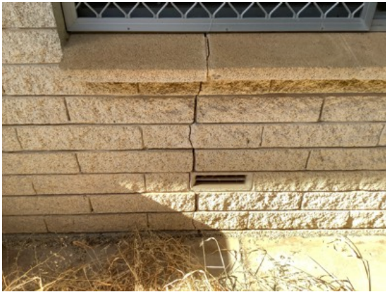
Vertical appearance cracking observed to the South elevation brick wall below the Meals area window. Recommend repairs and to monitor over time.
