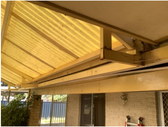
Significant damage, distortion and sagging observed at the West elevation Patio to fascia connection. Repairs, modification and/or removal is required to prevent further damage. and to make safe.
