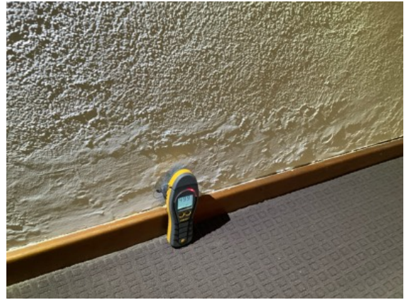
Moisture detected to the Lounge wall is located directly adjacent to the Bathroom shower recess.
