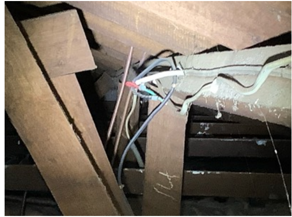
Exposed wiring junctions observed in the roof void above the Entry area. Recommend having an Electrician install junction box's at all connections to make safe.
