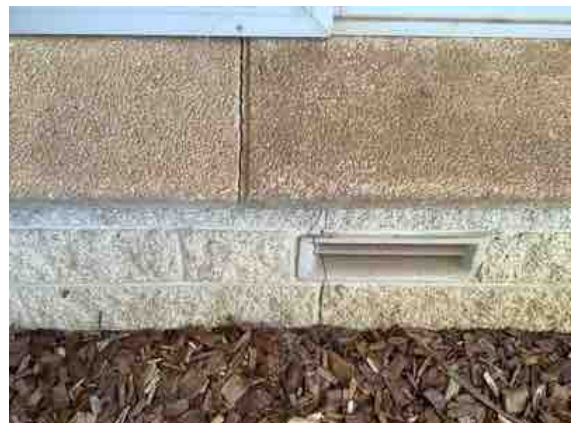
West elevation - Appearance cracking noted to the exterior brick wall below the Family Room window. Recommend maintenance/repairs and to monitor over time.
