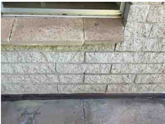
East elevation - Stepped appearance cracking noted to the exterior brick wall below the Bedroom 2 window. Recommend maintenance/repairs and to monitor over time.
