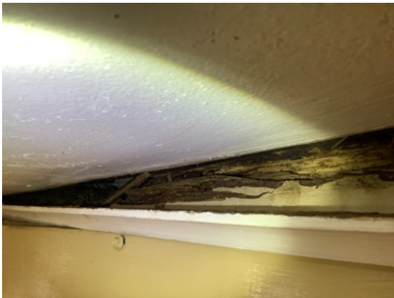
Significant wood rot damage noted to the exposed section of the timber Verandah beam. Recommend having Builder conduct an invasive inspection to the beam and roof frame to ensure there is no further concealed damage and repair as required.
