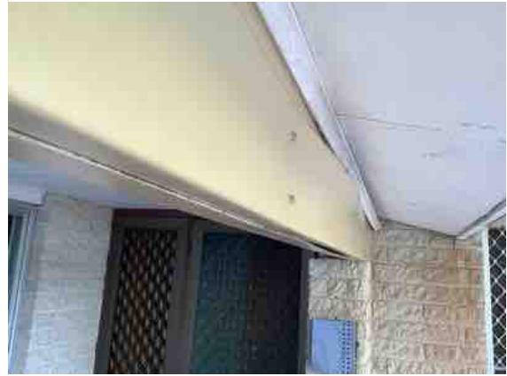
Distortion and buckling noted to the steel fitch plates installed to both sides of the Verandah beam which are failing to support the timber beam as intended. Repairs required.
