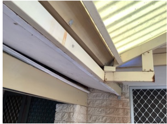
The West elevation Patio structure is connected to the metal fascia of the main residence only which is not designed to take load and has caused sagging and damage to the fascia gutter and eaves. Repairs, modification and/or removal is required to prevent further damage. and to make safe.
