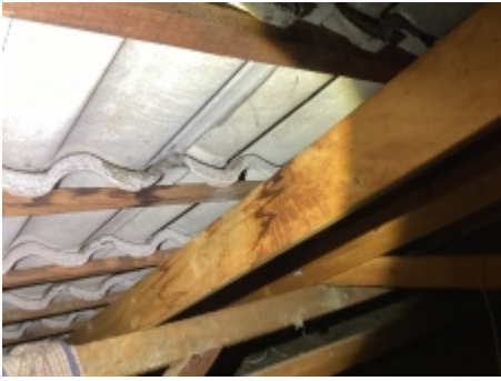
Showing examples of the moisture stains in the roof
