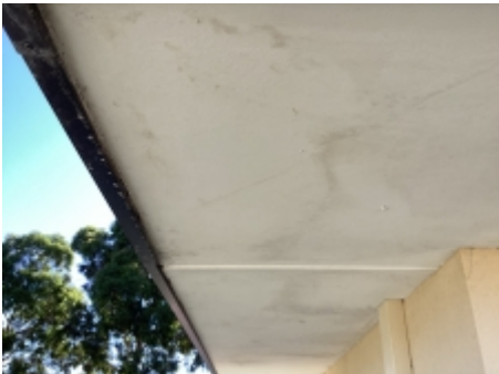
Showing examples of the moisture stains
