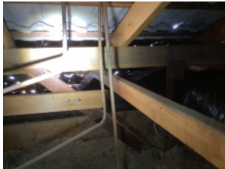
The major defect as observed constitutes a structural defect to the requirements of AS 4349.1-2007, Collar tie not installed correctly recommend builder to investigate further and repair as required
