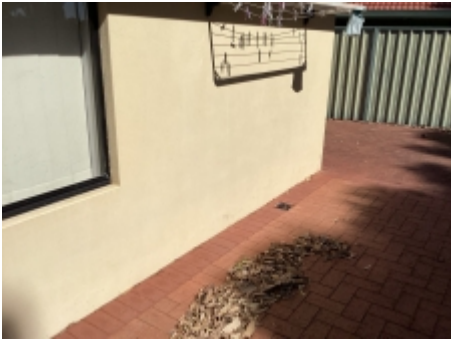
Showing examples of the covered weep holes
