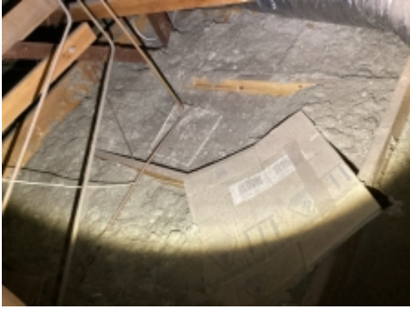
Showing examples of the moisture stains in the roof
