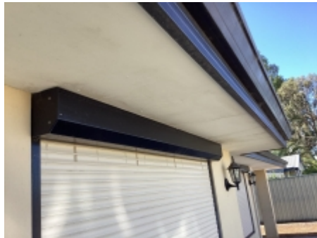
Showing examples of the moisture stains
