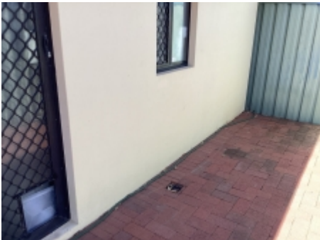
Showing examples of the covered weep holes
