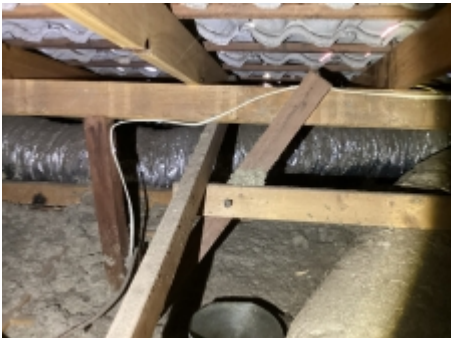
The major defect as observed constitutes a structural defect to the requirements of AS 4349.1-2007, Collar tie not installed correctly recommend builder to investigate further and repair as required
