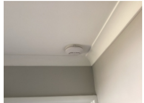
Showing examples of the smoke alarms
