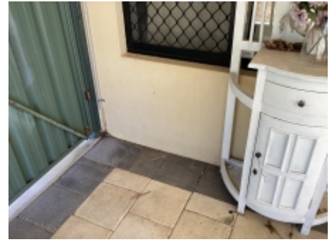
Showing examples of the covered weep holes
