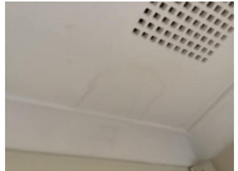
Showing examples of the moisture stains
