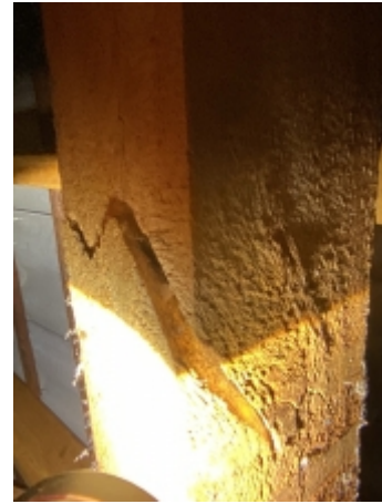
The major defect as observed constitutes a structural defect to the requirements of AS 4349.1-2007, Under purlin has cracked recommend engaging a builder to investigate further and repair as required
