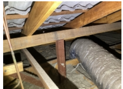
Showing example of insulation and AC duct to the ceiling space, Showing example of framing and low clearance in the roof space
