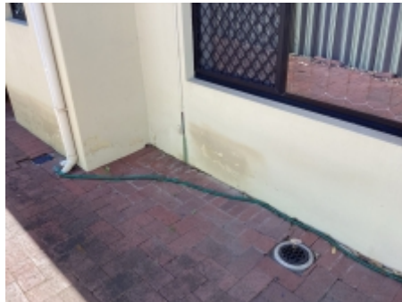
Showing examples of the covered weep holes
