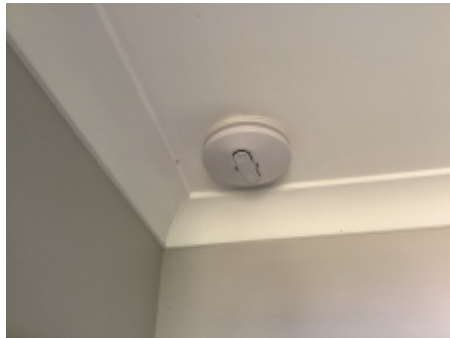
Showing examples of the smoke alarms
