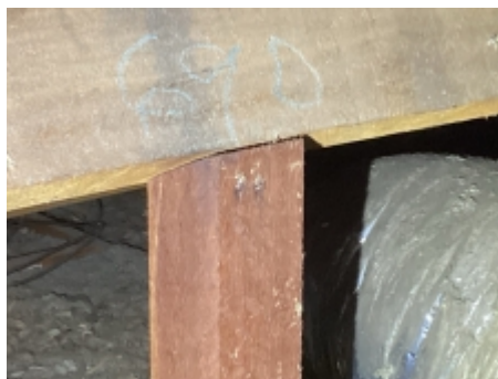
The major defect as observed constitutes a structural defect to the requirements of AS 4349.1-2007, Under purlin observed to be moving recommend builder to repair
