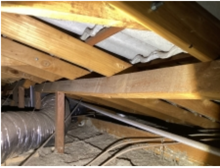
The major defect as observed constitutes a structural defect to the requirements of AS 4349.1-2007, Under purlin has cracked recommend engaging a builder to investigate further and repair as required
