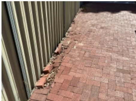
Showing undulating/uneven path
