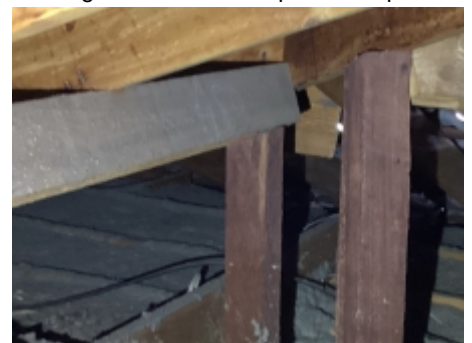
The major defect as observed constitutes a structural defect to the requirements of AS 4349.1-2007, Under purlin observed to be moving recommend builder to repair
