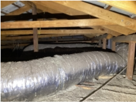
Showing example of insulation and AC duct to the ceiling space, Showing example of framing and low clearance in the roof space
