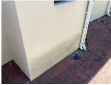
Showing examples of the covered weep holes
