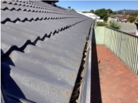
Showing examples of the debris in the gutters
