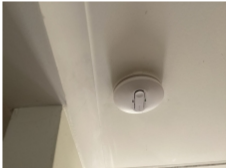
Showing examples of the smoke alarms
