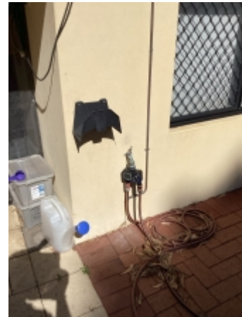
Showing examples of the covered weep holes
