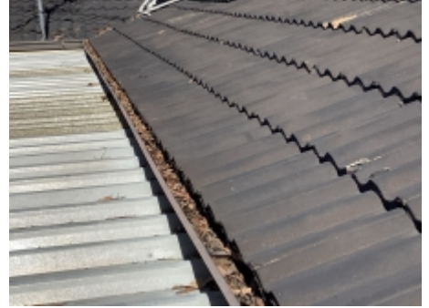
Showing examples of the debris in the gutters
