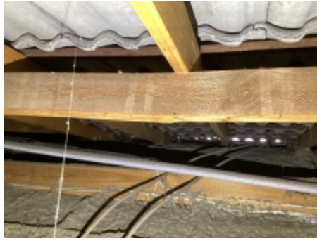
The major defect as observed constitutes a structural defect to the requirements of AS 4349.1-2007, Under purlin has cracked recommend engaging a builder to investigate further and repair as required
