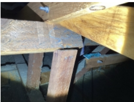
The major defect as observed constitutes a structural defect to the requirements of AS 4349.1-2007, Under purlin observed to be moving recommend builder to repair
